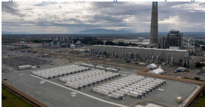
Figure 38: PG&E Moss Landing Tesla Battery Storage
