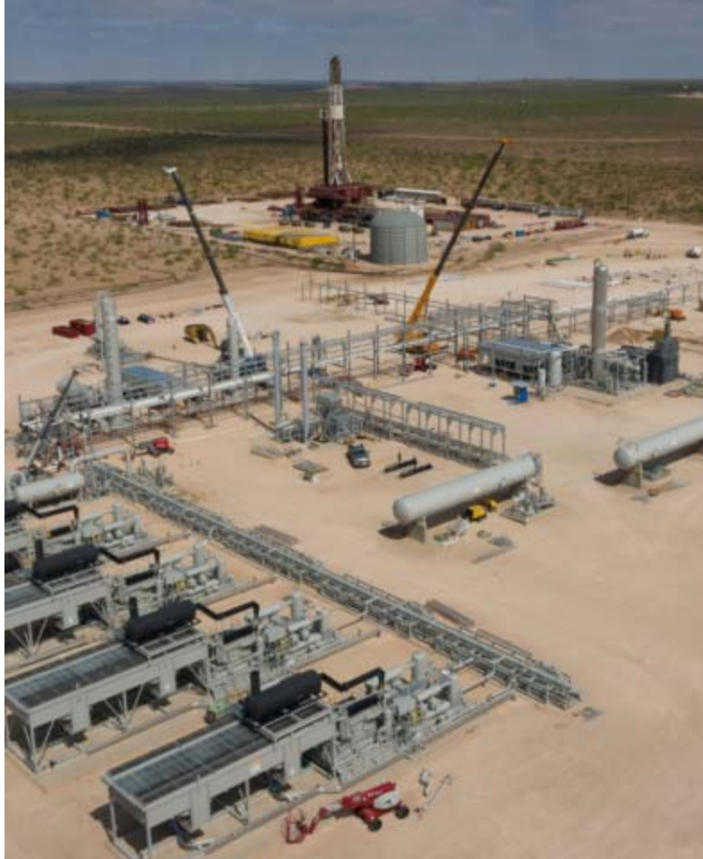
Dark Horse Amine Treatment and Carbon Capture Facility. Source: Piñon Midstream
